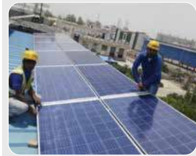
55kW p Installation, Kundli Industry/Sector : Engineering
