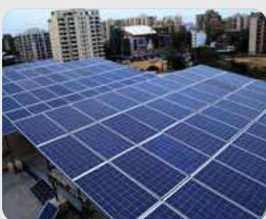
35kW p Installation, Gurugram Industry/Sector : Corporate Office
