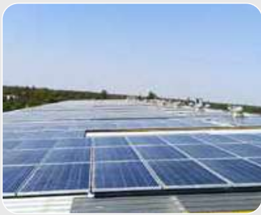
330kW p Installation, Jaipur Industry/Sector : Stone
